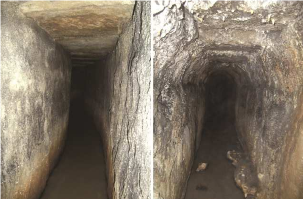
Figure 2: Different cross sections in the tunnel, left showing the tunnel path curved
