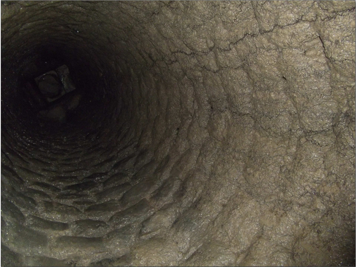
Figure 3: Dullab Shaft well in the tunnel ca. 100 m to the east from the tunnel entrance (looking upwards)
